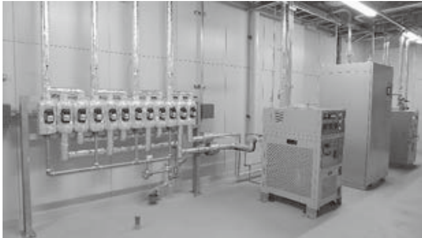
Photo 6 Machinery room with a nitrogen generator and a temperature/RH control system (② in Figure 2) (Image by the author, February 14, 2014)
