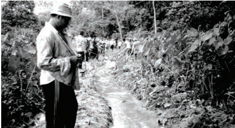
Plates 15 & 16: Gotong royong work along the Sedoi River . When the Sedoi River became clogged, the villagers came together to carry out drainage and irrigation work. They wore long-sleeved shirts with hats to protect them from the strong direct sunlight. [NT-1998]
