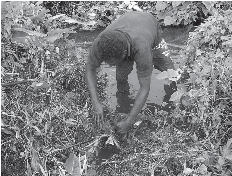
Figure 3 Eli Field Malau from Vētuboso village is repairing a water channel (photo at Rotluō, 2007)
