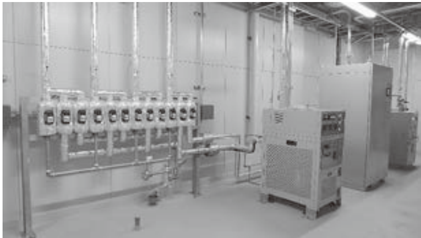
Photo 6 Machinery room with a nitrogen generator and a temperature/RH control system (② in Figure 2) (Image by the author, February 14, 2014)
