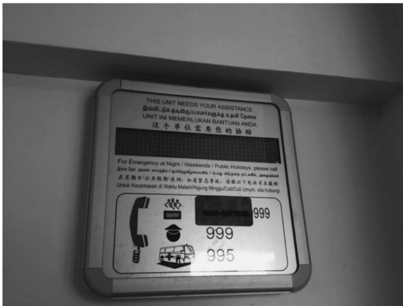
Photo 3 An Emergency Board
